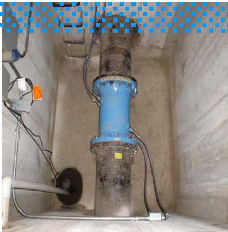
16" (DN400) 93C measures bi-directional flow in the vault of a water tower in Oswego, Illinois USA
