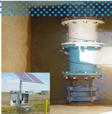
12" (DN300) 93C measures river water intake in Beaumont, Texas USA. 4-20mA signals are transmitted via wireless solar panel system from several remote locations.
