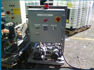
Ciba® ALCOTECH® LPU liquid polymer makedown unit in operation at Fon du Lac project
