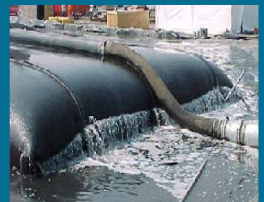
Filtrate flowing from geotube after slurry solids flocculated with Ciba ® KRYVALIS ® flocculant
