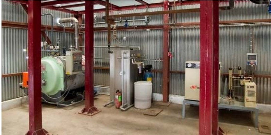
Fig. 6: Gas boiler system installed into the PSA desalination building
