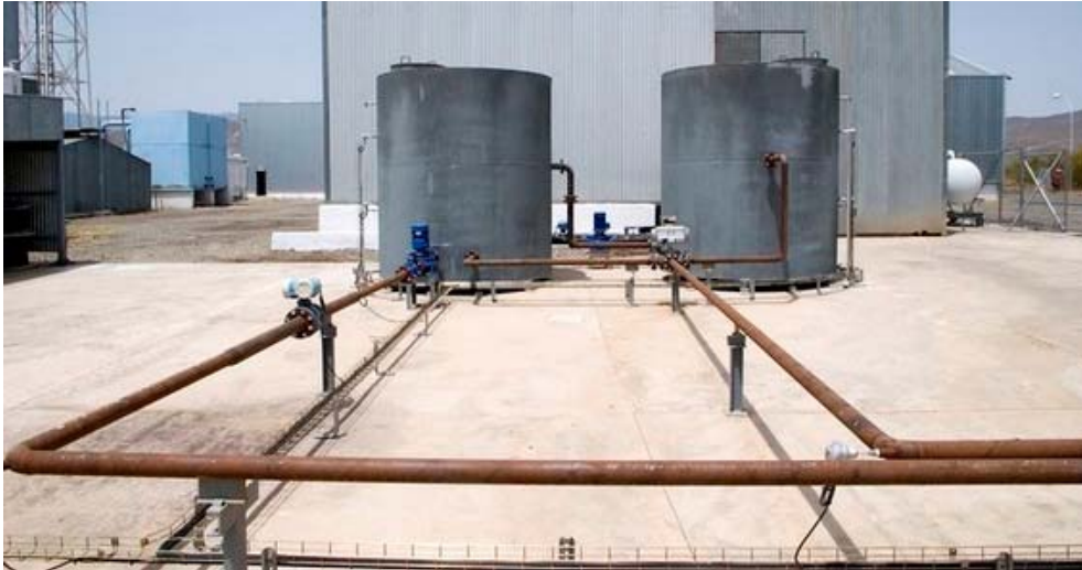
Fig. 5: Front view of the PSA desalination building with the two thermal storage tanks
