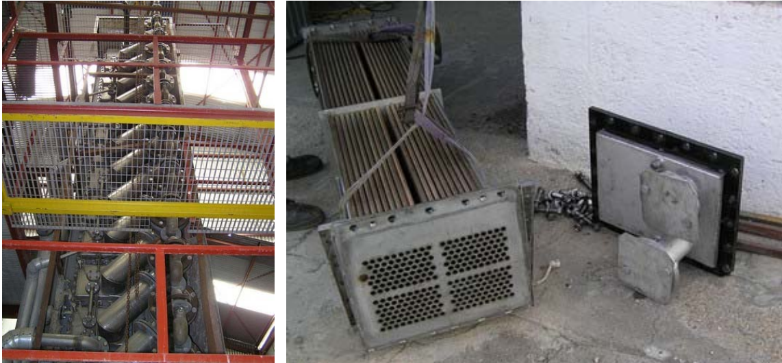
Fig. 2: The PSA MED plant (left) and the new horizontal tube bundle installed at the first effect (right)
